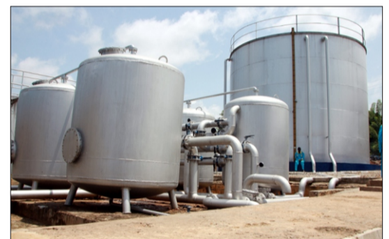
Water treatment plant at Okemesi
