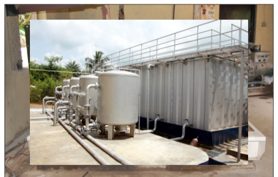
Water treatment plant at Ido Ile
