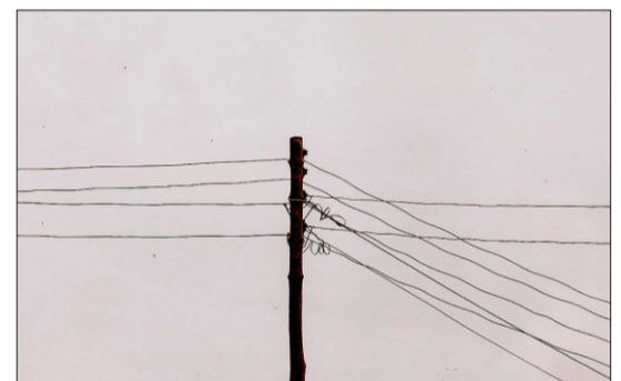
Electricity extension at Araromi, Ipoti.
